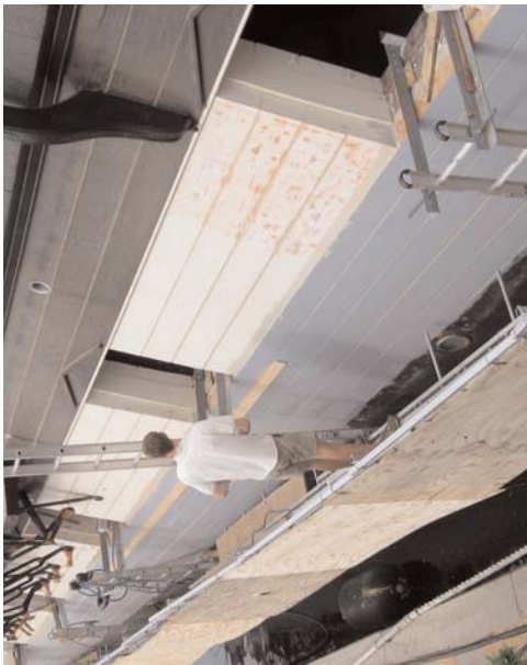
Repair work on Constellation's hull continues. The photo shows that the outer layer of planking has been primed, ready for finish coat.
