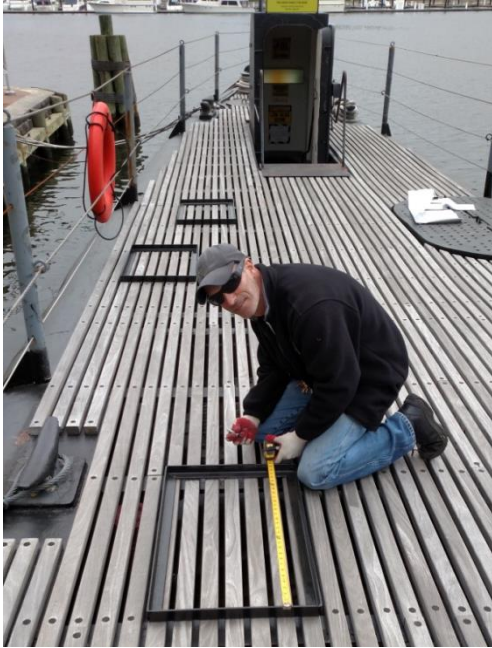
Pier 3 Manager Rob Howard measures a section of the main deck on USS Torsk while planning for the installation of several removable deck hatches.
