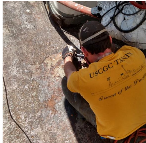
Pier 5 Manager Ryan Szimanski uses a pneumatic piston scaler to clean a portion of USCGC Taney's starboard main deck to bare metal for repair and painting.
