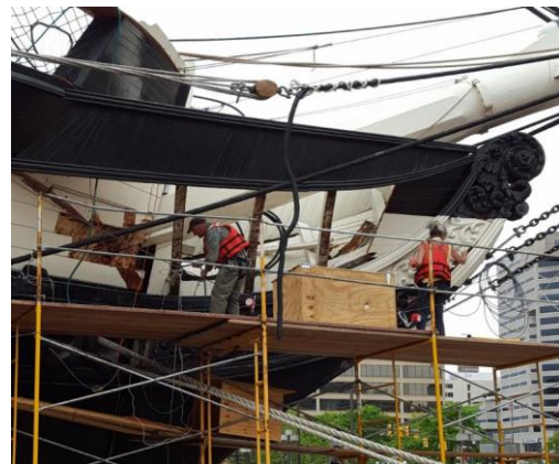
Pier 1 Manager Tim Fowler and Constellation Shipwright Joan Murphy repair the beak of USS Constellation .
